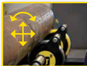
Alignment, side shift, and leveling functionality.
